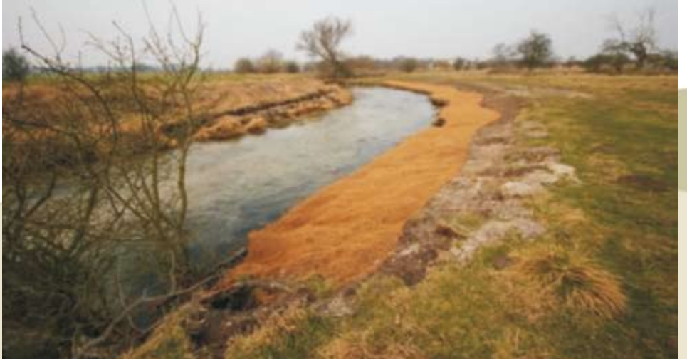
Once filled, the friable soil was protected by using a coir geotextile. The area will be allowed to recolonise with natural plant species.
