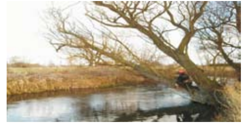
Removal of dangerous limbs from a riverside tree. These limbs were used as in-channel habitat and securely pinned to the riverbed. Small coarse material from these limbs was used to protect the 'toe' of vertical banks and provide habitat for voles, fry and kingfishers.
