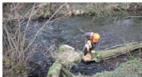
A felled alder being prepared for anchoring to its original tree stump.
