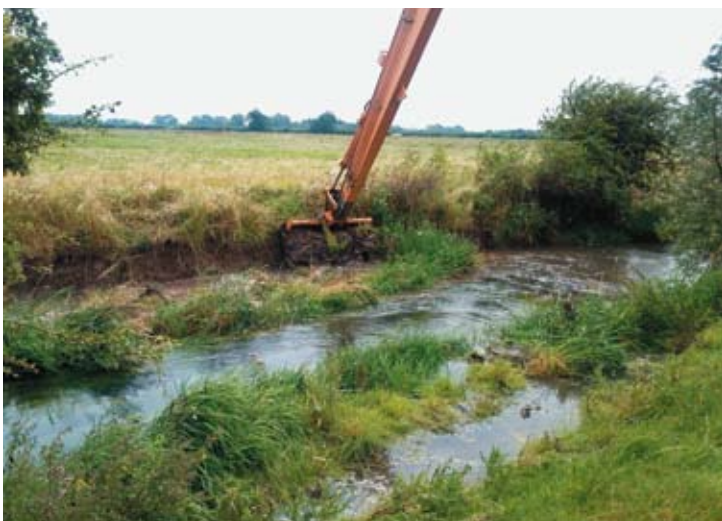
The long-reach excavator at work re-profiling the far bank and using the material to backfill the void left after dragging the reed beds into the stream to narrow up the channel
