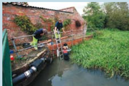
Installation above the gauging weir. View of the pass header box with the engineers fitting the cables and pipes to supply water to the pass
