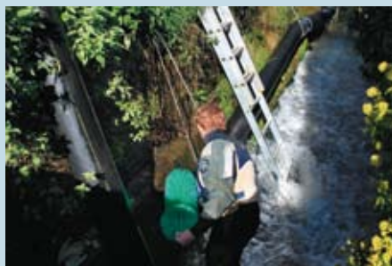
As each section of pipe was installed the media was inserted that would enable the eels to move through the pass
