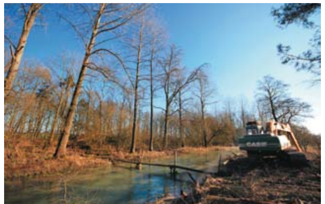
The Environment Agency provided this 22 tonne excavator to position heavy logs in the stream
