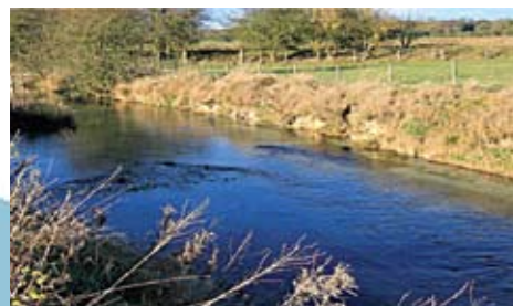
View looking at the top of the site showing erosion to the left bank
