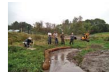
Volunteers assisting with works - coir logs installed on outside of 'new' meander
