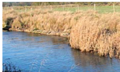
Bank toe protection using coir rolls. The rolls are staked and backfilled to promote natural plant growth from seeds present in the river sediment
