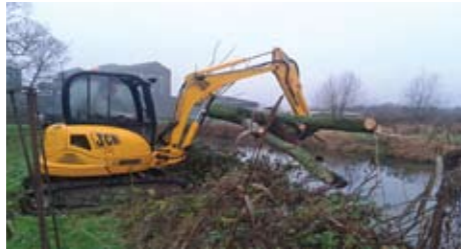
Placing a large log close to the left bank as a deflector. A total of nine such structures were positioned through the project site. These logs were drilled and pinned to prevent any movement
